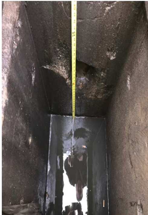
Photo 1 – Catch basin after a winter of treated salt usage on area roads. The sump remains empty of debris and only melt water is left.
