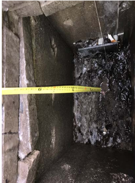
Photo 2 - Catch basin that was not cleaned since the change to treated salt.
